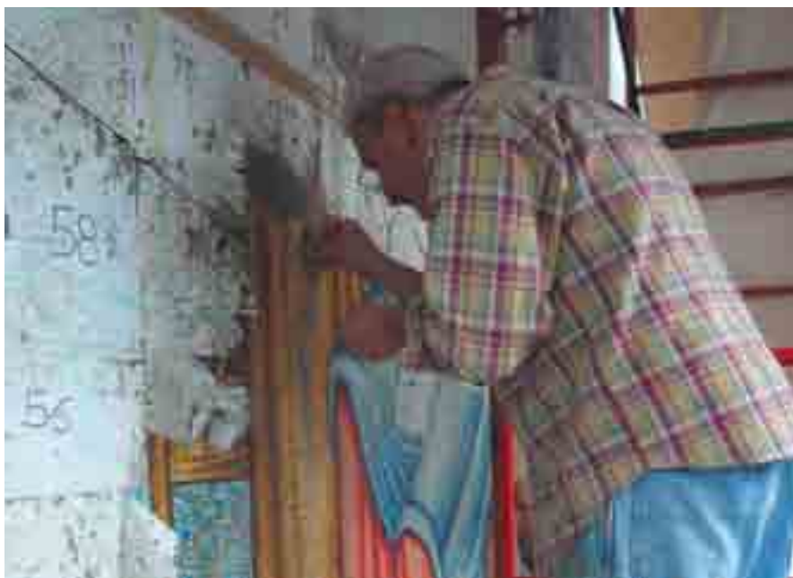
CUSTOM CRAFTWORK To install the massive mosaic at Holy Family Catholic Church in Stow, Radiant Art co-owner Jim Foltz works from the center outward, attaching tiny Venetian enamel mosaic tiles to the wall using latex-based cement mixtures.
